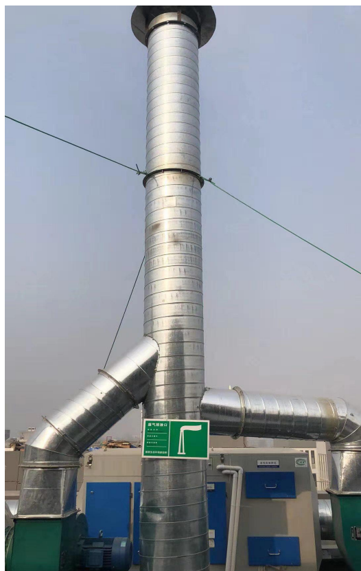
废气排放口标牌
